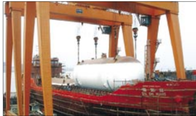
At its Taizhou shipyard, I.M. Skaugen installs a cargo tank on the second Summargas vessel, a 3,200 cu m pressurized LPG vessel, "Qin Shi Huang". The vessel was delivered to its owner in February 2008.
